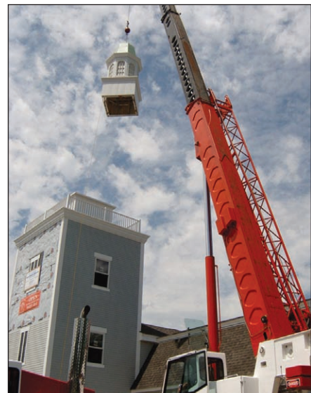
A crane hoists the cupola from the New Hampshire Antique Co-op into place.
